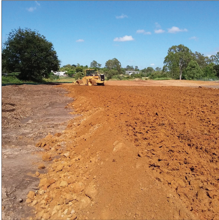
Figure 5. Compactor used throughout bulk earthwork activities to spread and compact material. (Taken 04/02/2021)
