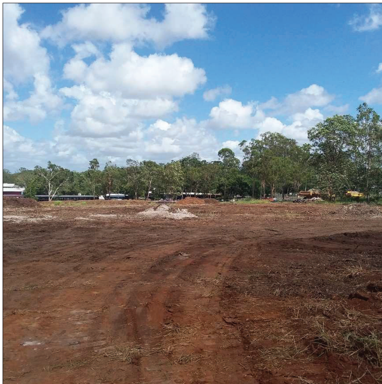
Figure 2. Post-strip inspection (Taken 28/01/2021)
