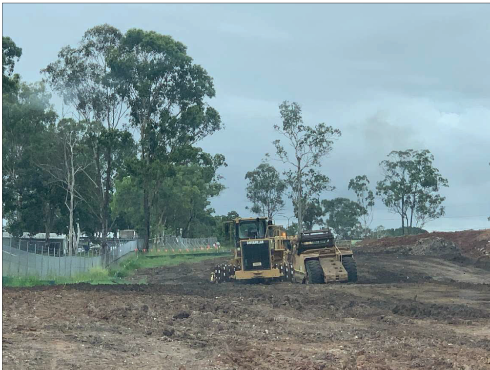
Figure 6 – Compactor and scraper working in conjunction to spread and compact material. (Taken 10/02/2021)
