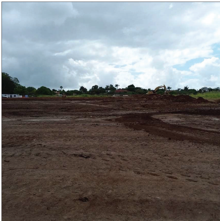
Figure 4. Post-strip inspection (Taken 01/02/2021)
