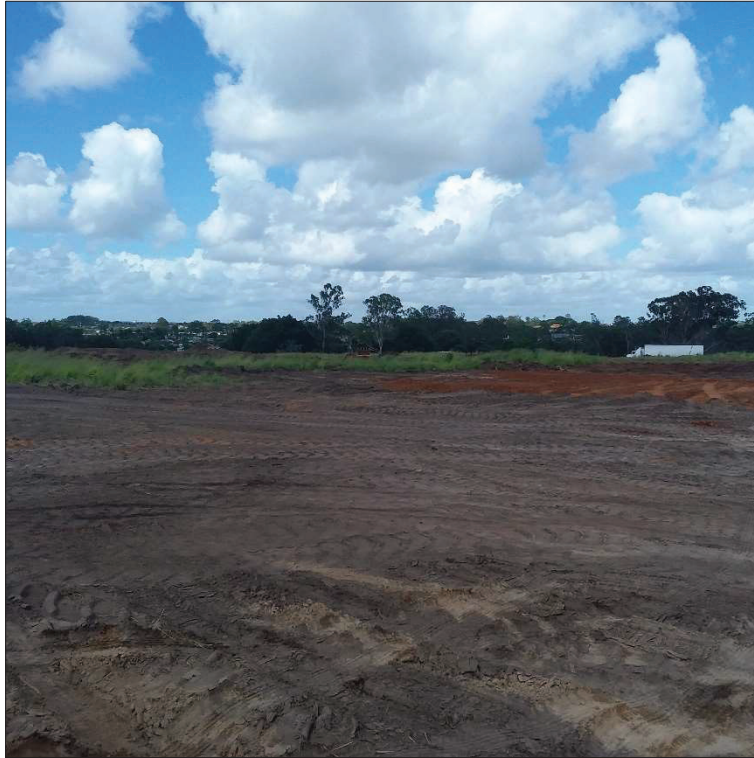
Figure 3. Post-strip inspection (Taken 28/01/2021)
