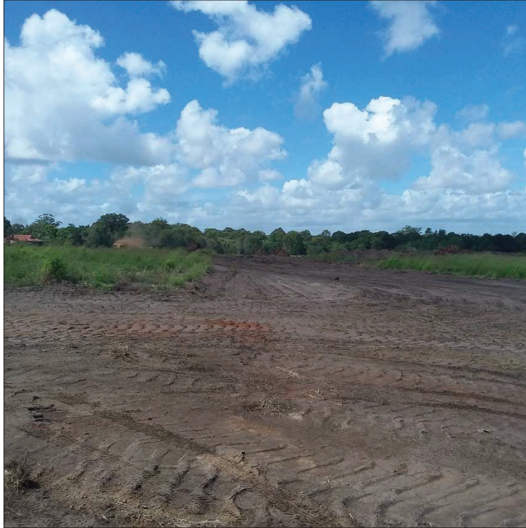
Figure 1. Post-strip inspection (Taken 28/01/2021)
