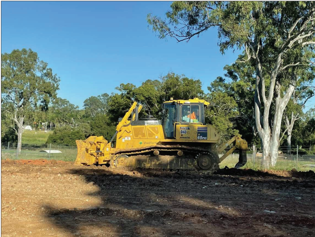
Figure 17. Dozer used throughout bulk earthwork operations to cut and spread material. (Taken 20/04/2021)
